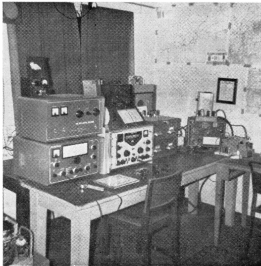
Neat Hq. station of the Royal Naval Amateur Radio Society, G3BZU, at H.M.S. "Mercury," near Petersfield, Hants. Equipment consists of a K.W. Viceroy SSB transmitter with matching Linear PA (these being the two items on the left), a Racal RA-17 receiver, a BC-221 frequency meter, and all the necessary ancillaries. The main operating schedule is 1230-1315 and after 1830 daily on 3720 kc, and Wednesdays are devoted to DX on 14 mc. AM/CW/SSB can be worked in the appropriate section of any HF band, and contacts are looked for with AT station operators interested in the Royal Navy.
